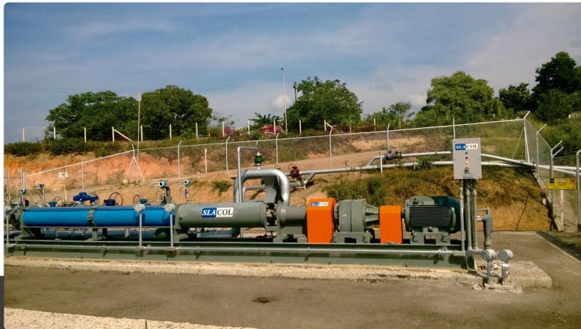
Multiphase surface pumping system
